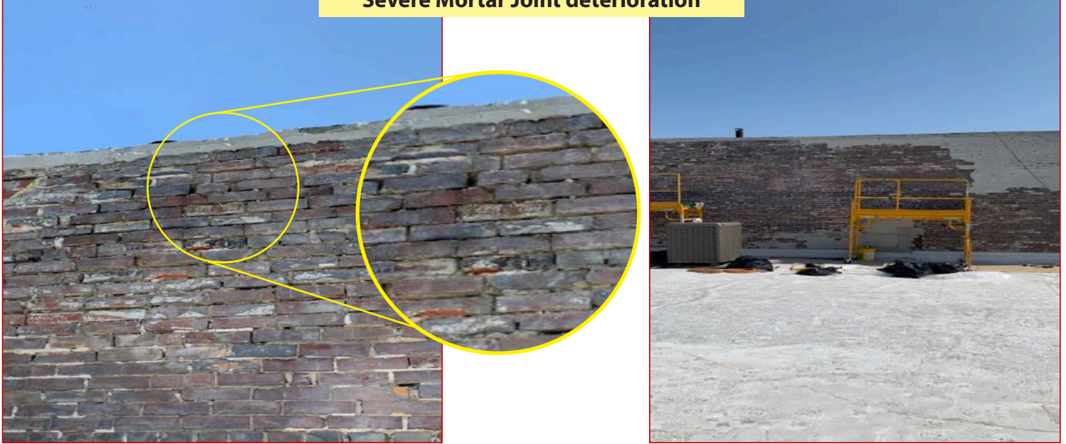
Severe Mortar Joint deterioration
